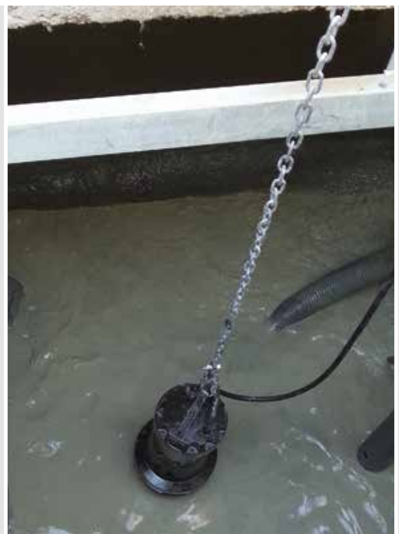
Pumping system for treated water for use in irrigation (Ireland) Two ZUG HP 050A 9/2 AW pumps
