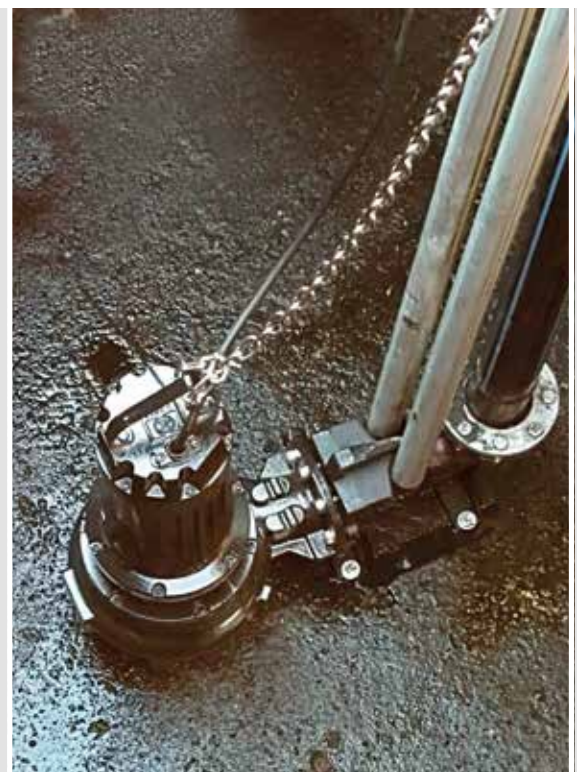
Lifting station pumping rainwater from collection tanks (Italy) Four ZUG V 100B 5.5/4 AW pumps
